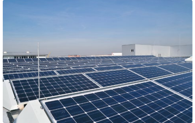
Rooftop PV panels at Tamron Europe GmbH
