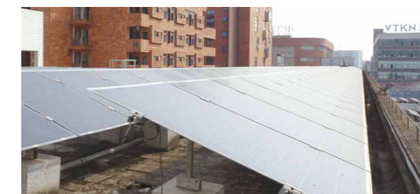
Solar power generation system (improvement at Foshan plant, China)
