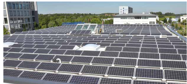
Solar power generation system (improvement at Tamron Europe)
