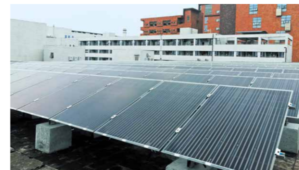
Solar power generation system (improvement at Foshan plant, China)
