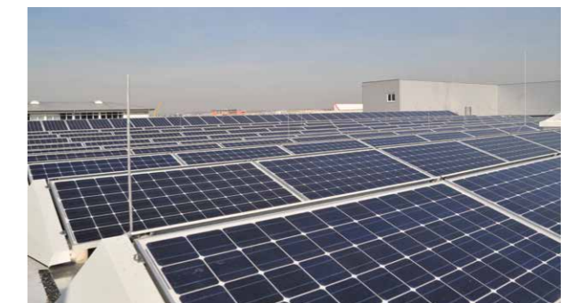
Solar power generation system (improvement at Tamron Europe China)
