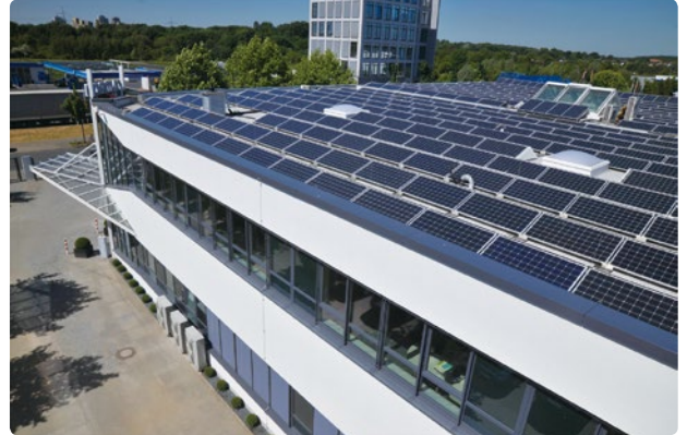
Rooftop PV panels at Tamron Europe GmbH
